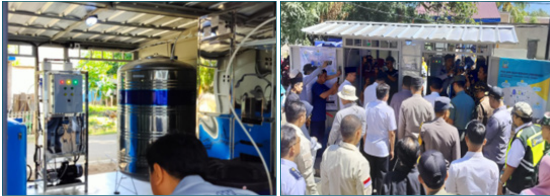
FIGURE S.10 SWRO water treatment plant
